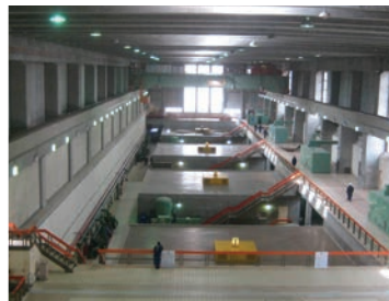
Kpong, Ghana 160 MW Rehabilitation of the second largest hydroelectric dam in Ghana
